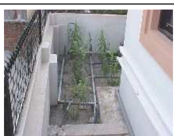
Figure 57 Reed bed for Gray Water Treatment
