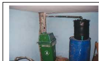
Figure 56 Urine and Faeces Collection by means of polythene tanks
